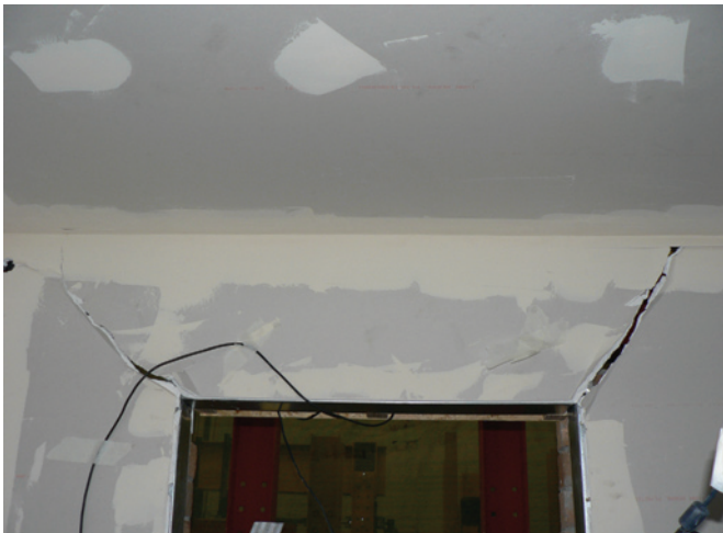
Internal lining damage at maximum load.
