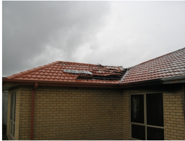
Figure 6: Hole in the roof from the East Elevation of the house
