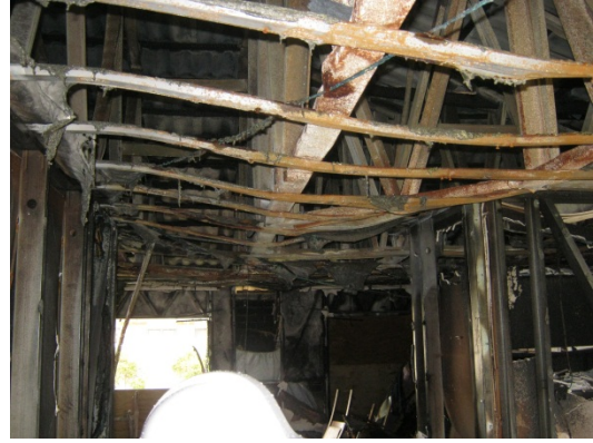
Figure 2: Living room showing distortion of the steel roof trusses and ceiling battens
