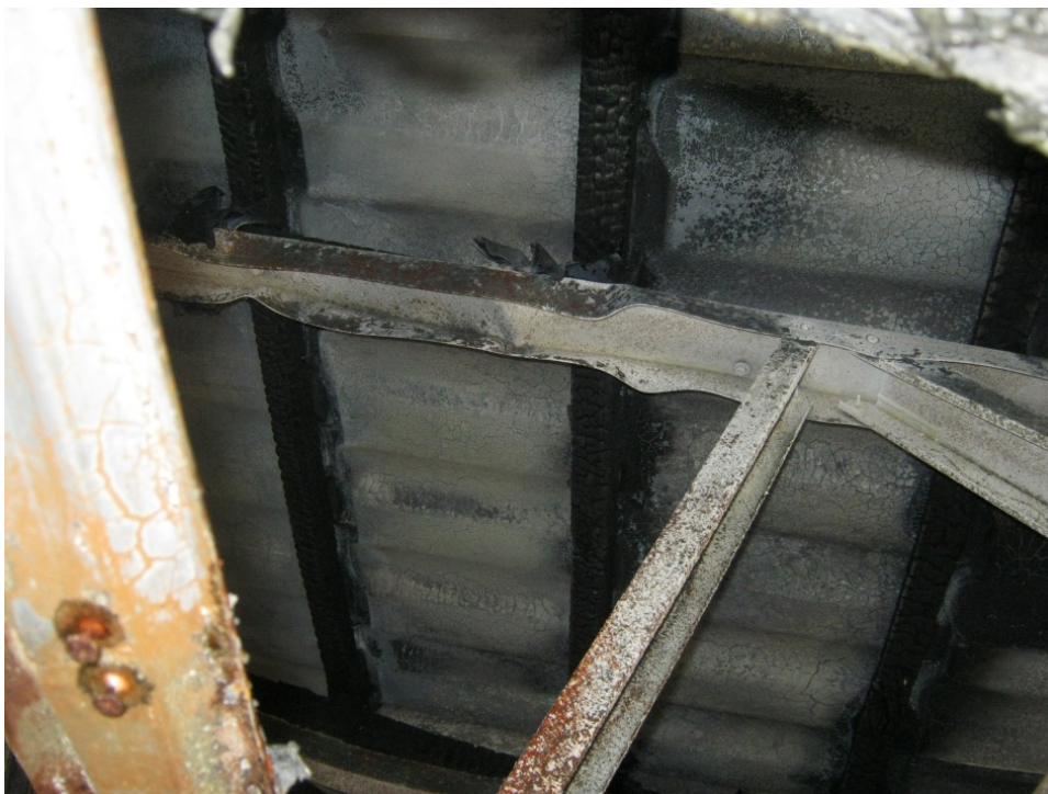
Figure 14: Image showing the charred battens
